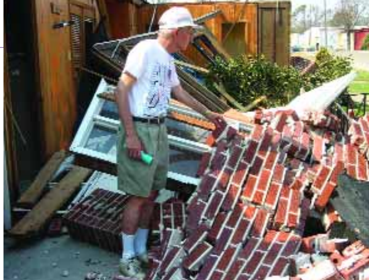
Rev. Adam Cooper looks over the damage at the fellowship hall at St. Matthew Lutheran Church in Gulfport, Miss. The sanctuary suffered only minor roof damage, but the foyer of the fellowship hall was destroyed. Rev. Cooper was planning on retiring in January, but is rethinking his plans in view of the overwhelming losses of many of the church's members.
